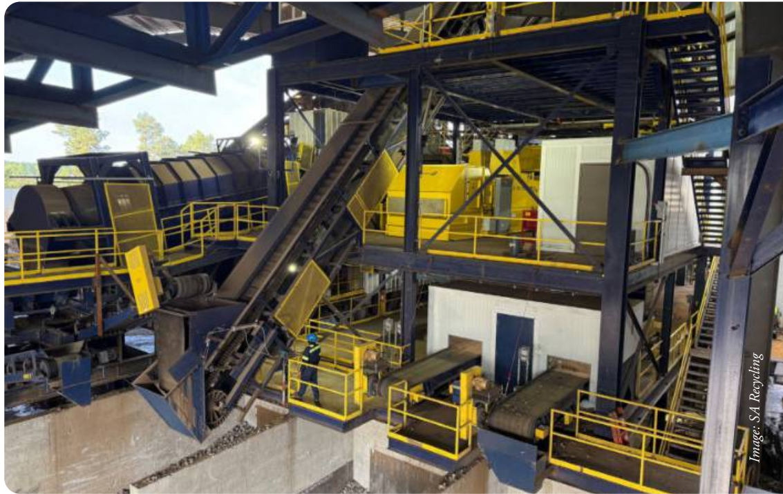
Sensor sorting plant to make high-grade aluminum such as vesper in Atlanta, GA
